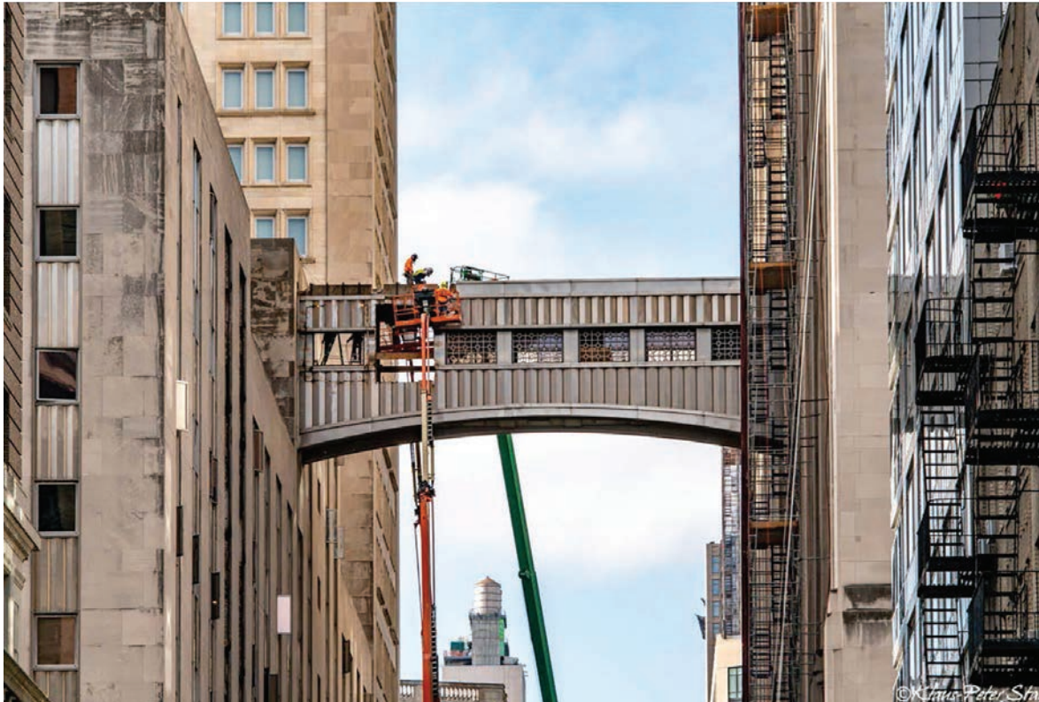
Another unheralded demolition in 2020: an undesignated skybridge at East 24th Street. It connected portions of the MetLife campus. Photo: Klaus-Peter Statz for Untapped New York. But not only skybridges are disappearing.
