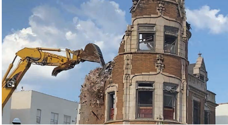
The demolition of the Dangler House as seen in an NBC News video.
